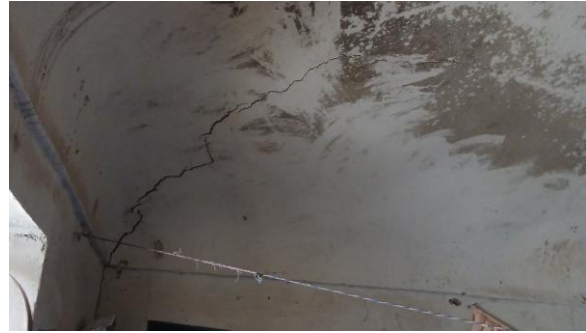
b) Vertical crack that separates the in-plane and out-of-plane walls at the corner, which also extends to the vault roof during the 2023 Herat earthquake.
