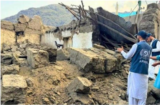
c) The mud wall and wooden roof collapsed during the 31 August 2025 earthquake in eastern Afghanistan 1 .
