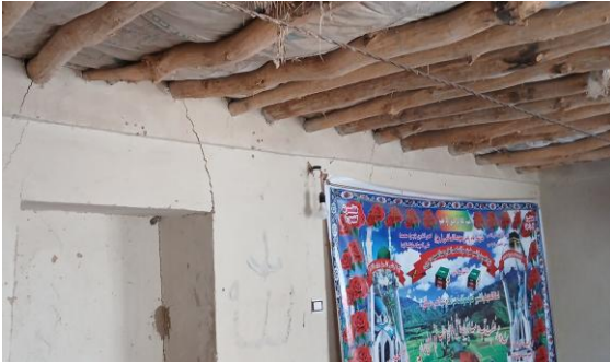
a) Diagonal cracking in an adobe masonry wall caused by lateral stresses and weak roof-wall connections in a traditional timber log roof system during the 2023 Herat earthquake.
