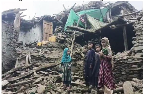
e) Dry stone walls collapsed in the 31 August 2025 earthquake in Kunar Province, eastern Afghanistan 3 .
