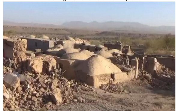
f) Arch ceiling damage caused by the 7 October 2023 earthquake in Herat Province, Afghanistan 4 .
