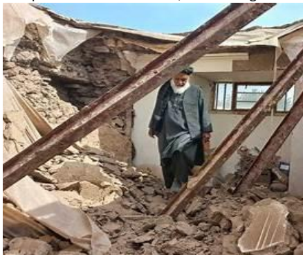
g) Collapse of a house with steel roof girders in Herat Province following the October 2023 earthquake 5 .
