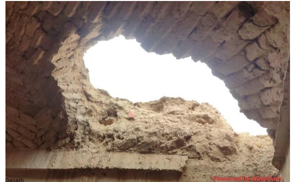
d) Partial damage to the thick vault roof made of mud bricks during the 2023 Herat earthquake 2 .
