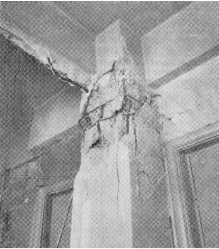
Bending damage at upper end of a column in a block with partial collapse (see Balan, 1980: Figure VI.19:b. on page 246)
