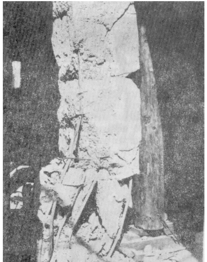
Ground floor column, destroyed due topounding with neighbouring building (see Balan,1980: figure VI.20.d. on page 247)
