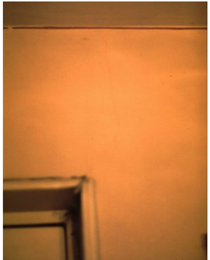
Vertical rift in shear wall going out
