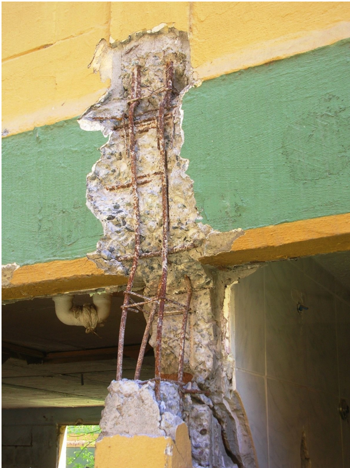
Improper detailing of tie-beam-to-tie-column joint
