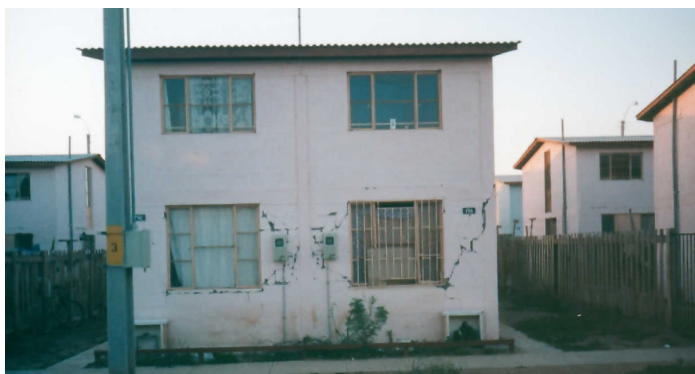
Photograph illustrating typical earthquake damage (1997 Punitaqui earthquake)
