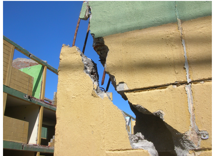
Shear failure of tie-column
