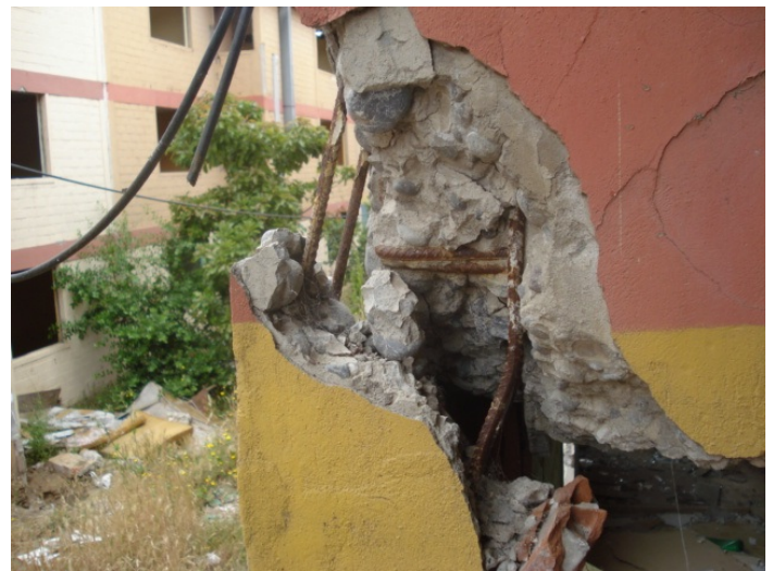
Absence of ties in the joint region
