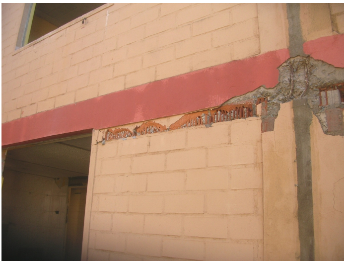
Out of plane cracking in the longitudinal wall
