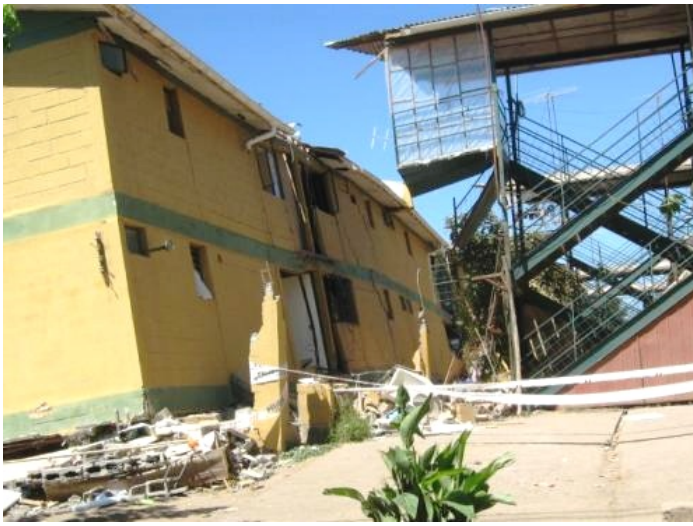
Collapsed three-story partially confined building in Santa Cruz, 2010
