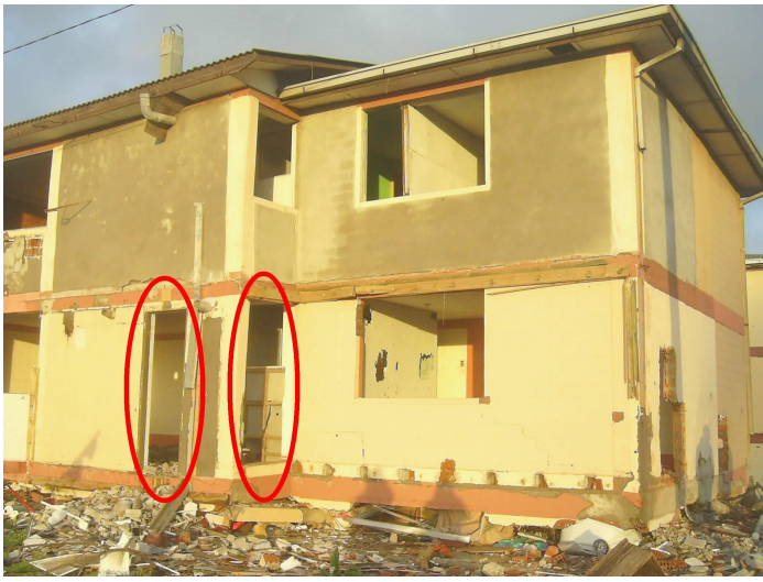
Collapse of building in construction, door opening at the second floor
