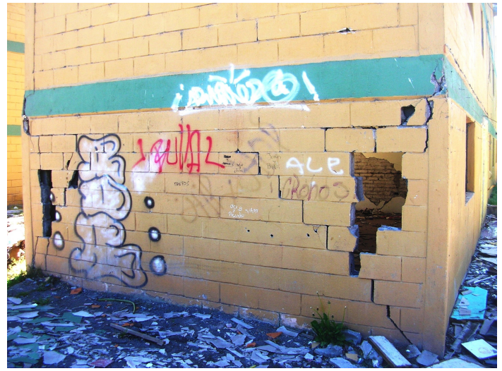
Stair-stepped cracking and masonry disintegration
