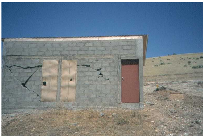
Earthquake damage (1997 Punitaqui earthquake)
