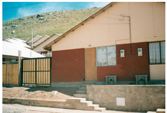
Earthquake damage (1997 Punitaqui earthquake)
