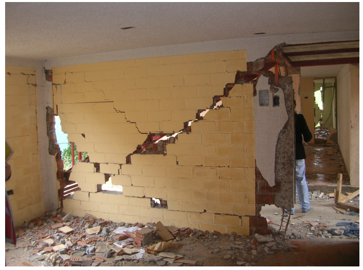
In-plane shear failure
