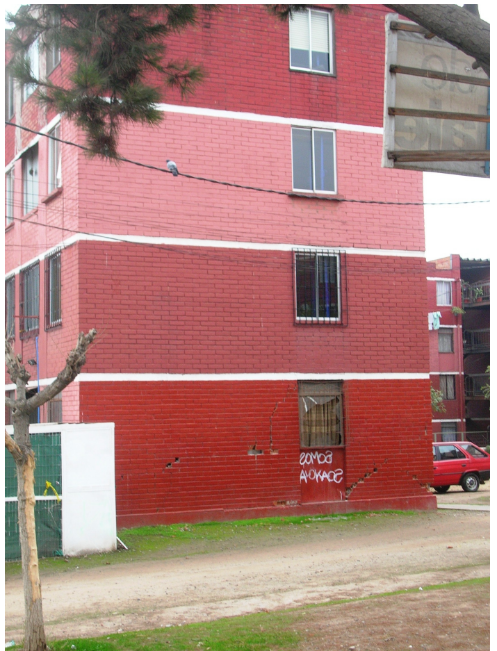
Unrepaired building with damage after 2010 earthquake. Conjunto Alberto Larraguibel. Comuna de Lo Prado, region Metropolitana
