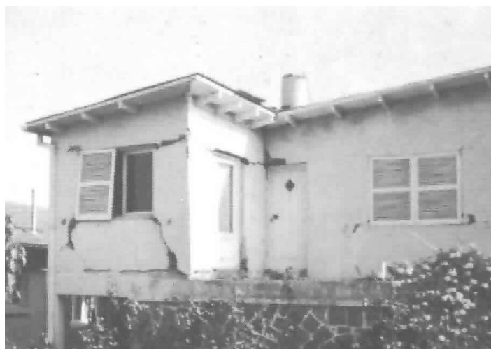
Typical earthquake damage: cracking of masonry walls (1985 Lilloe earthquake)
