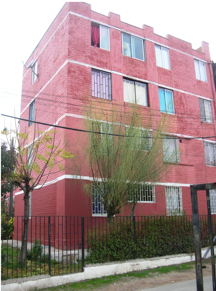
Building retrofitted after 1985 earthquake, without damage. Conjunto Alberto Larraguibel. Comuna de Lo Prado, region Metropolitana
