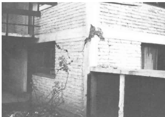
Typical earthquake damage: cracking of concrete posts and masonry walls (1985 Lilloe earthquake)
