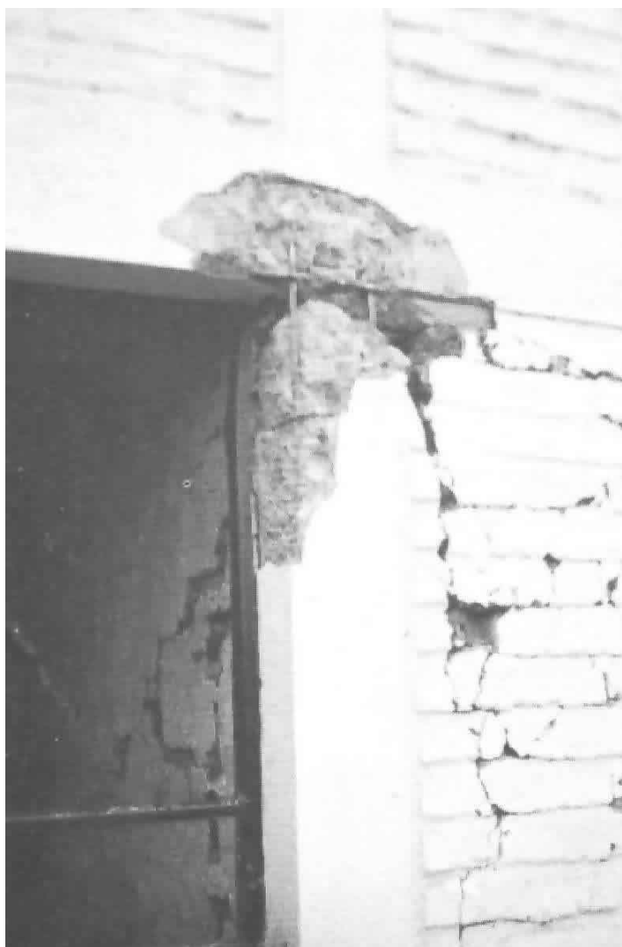
Typical earthquake damage: cracking of concrete posts (1985 Lilloe earthquake)
