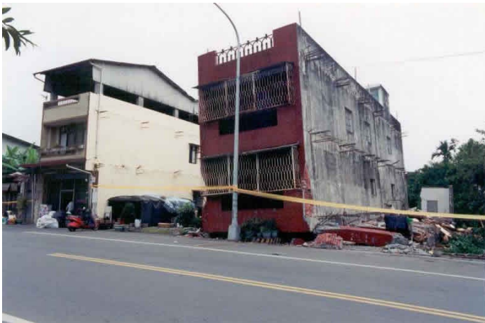
Earthquake damage - Collapsed Three-story building in the 1999 Chi Chi earthquake (Source: EERI 2001)
