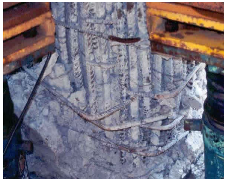
Earthquake Damage - Opening of 90 degree column hooks in the 1999 Chi Chi earthquake (Source: EERI 2001)
