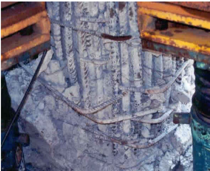
Earthquake Damage - Opening of 90 degree column hooks in the 1999 Chi Chi earthquake (Source: EERI 2001)
