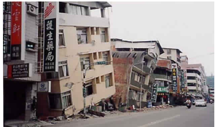
A Photograph Illustrating Typical Earthquake Damage (1999 Chi Chi earthquake)
