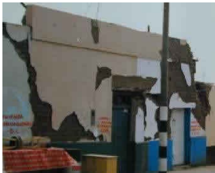
A Photograph Illustrating Typical Earthquake Damage (November 1996 Nasca Earthquake)
