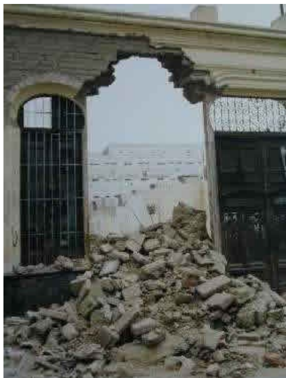
A Photograph Illustrating Typical Earthquake Damage (November 1996 Nasca Earthquake)
