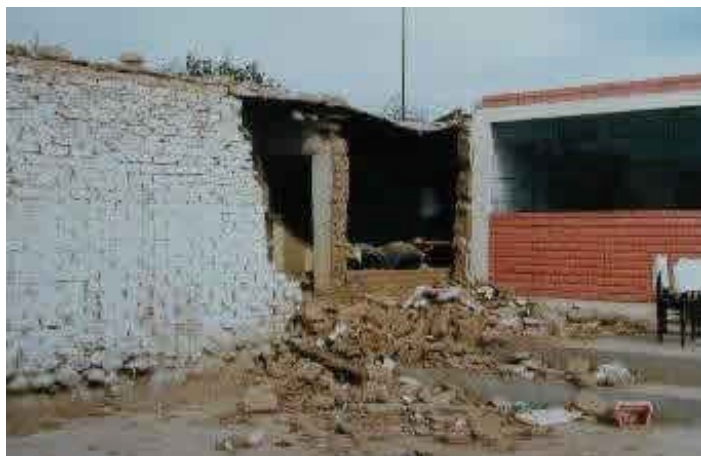
Key Seismic Deficiencies - Wall Damage Due to Inadequate In-Plane Seismic Resistance
