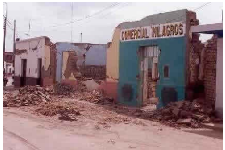
Key Seismic Deficiencies - Adobe Wall Failure Due to Out-of-Plane
