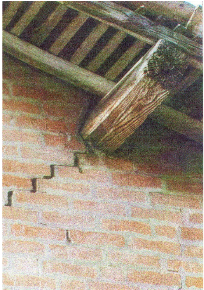
Wall damage at the roof beam support (1996 Bagnolo earthquake)
