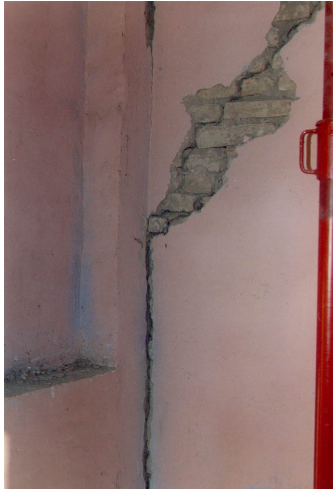
Seismic deficiency- inadequate wall connection
