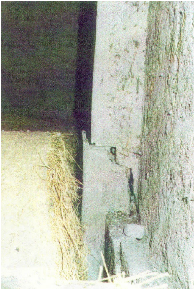
Wall damage (1996 Bagnolo earthquake)
