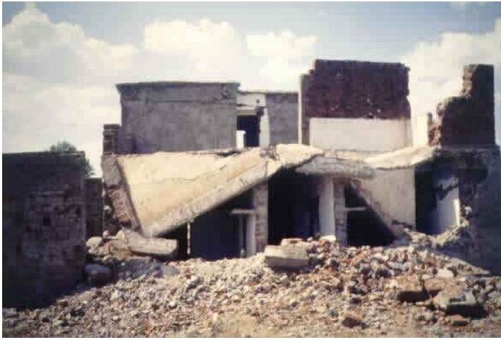
Typical Earthquake Damage - Roof Collapse Caused by the Wall Collapse (1993 Killari Earthquake)
