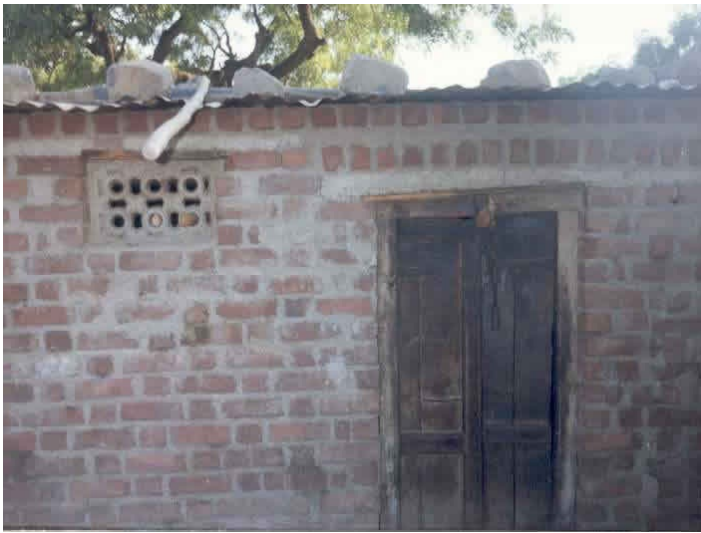
Construction Deficiency - Discontinuous RC Lintel Band
