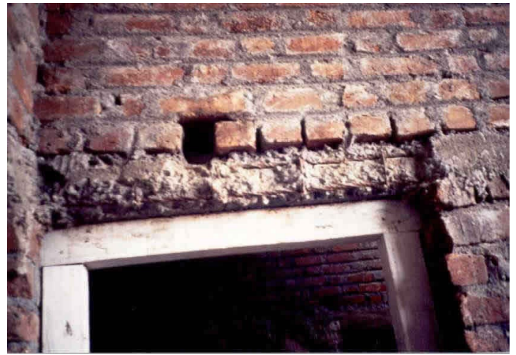
Construction Deficiency - Exposed Steel Reinforcement in RC Lintel Band Construction
