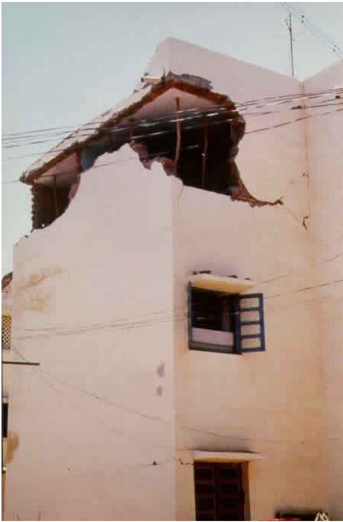
Partial Building Collapse in the 1997 Jabalpur Earthquake
