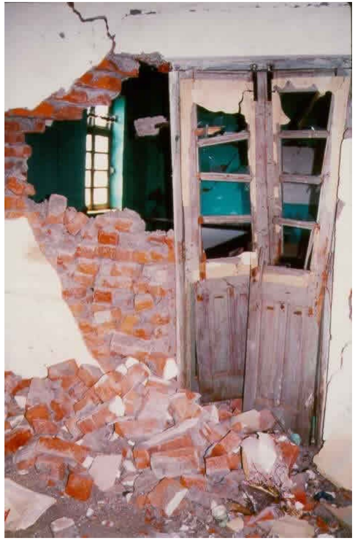
Failure of Brick Masonry Walls in the 1997 Jabalpur Earthquake
