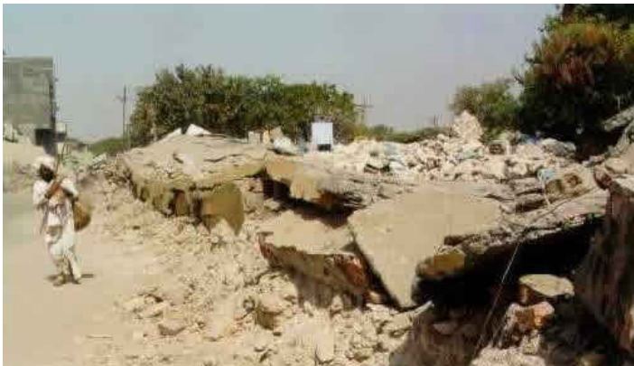
Collapse of Brick Masonry Buildings in the 2001 Bhuj Earthquake (Source: IIT Powai, 2001)
