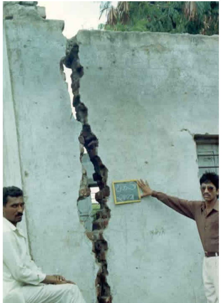
Typical Earthquake Damage - Wall Corner Failure (1993 Killari Earthquake)
