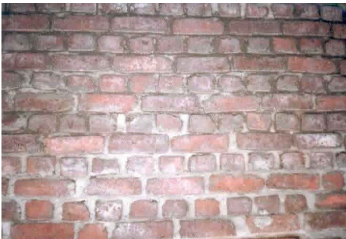
Construction Deficiency - Excessively Thick Mortar Bedding Joints
