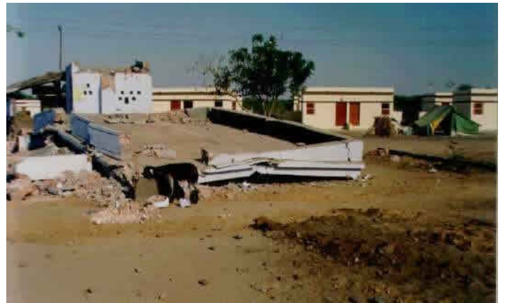
View of a Collapsed traditional brick masonry building in cement mortar (foreground) and masonry building with lintel bands which sustained only a moderate damage in the 2001 Bhuj earthquake (Source: IIT Powai, 2001)
