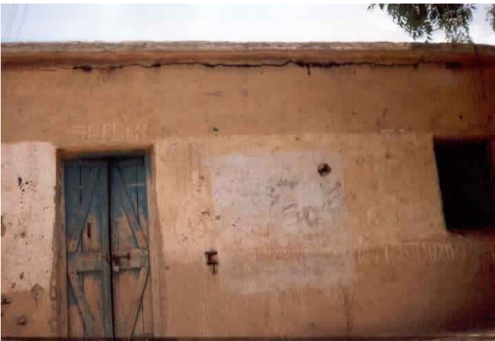
Typical Earthquake Damage - Sliding Failure of Roof-Wall Connection Due to the Absence of Wall Reinforcement (1993 Killari Earthquake)
