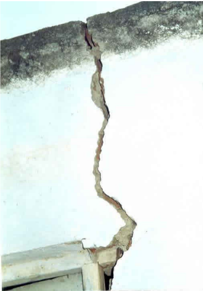
Typical Earthquake Damage - Wall Cracking above the Door Opening (1993 Killari Earthquake)
