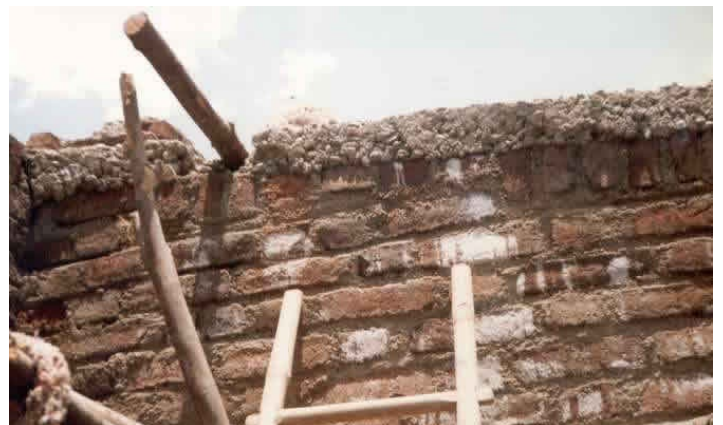
Construction Deficiency - Discontinuous RC Lintel Band (Bond Beam)
