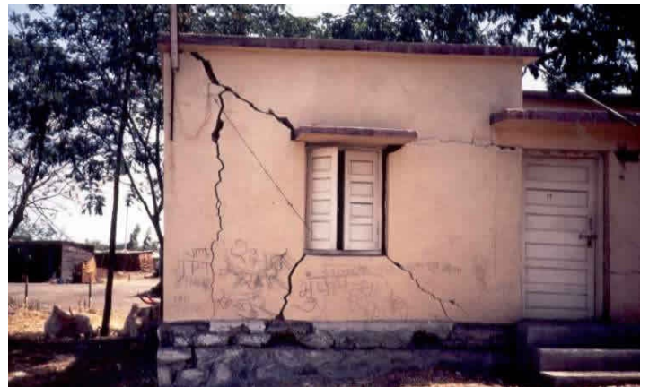
Typical Earthquake Damage: In-Plane Wall Cracking (1993 Killari Earthquake)
