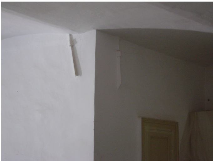
Figure 12. Old metallic tie
