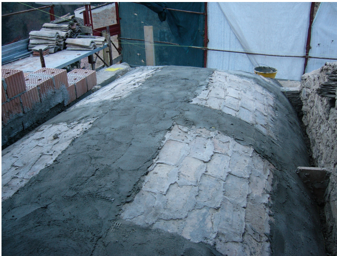
Figure 13. Vault restored covering the extrados with structural glass fibres and fixing it with their glues
