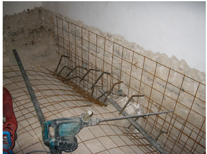
Figure 14. Vault restored covering the extrados with a welded mesh drown into a reinforced concrete overlay
