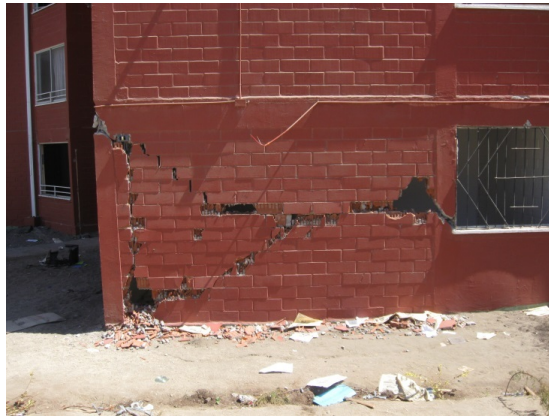
Figure 14. In-plane shear failure in buildings and shear failure at the ends of a reinforced concrete tie-column observed in 2010 earthquake in the city of San Antonio.
