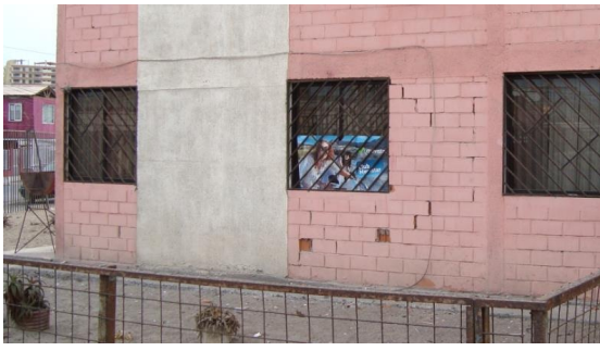
Figure 15. Damages of confined masonry buildings in the 2014 earthquake in the city of Iquique.
