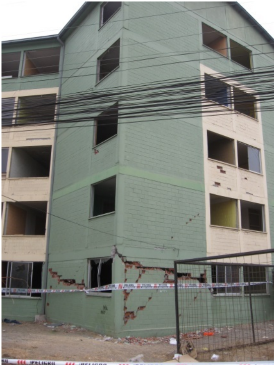
Figure 13. In-plane shear failure in buildings observed in 2010 earthquake in the city of San Antonio.
