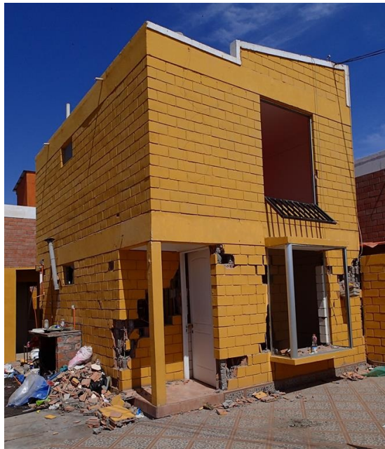
Figure 16. Damages of reinforced masonry houses in the 2014 earthquake in the city of Iquique.
