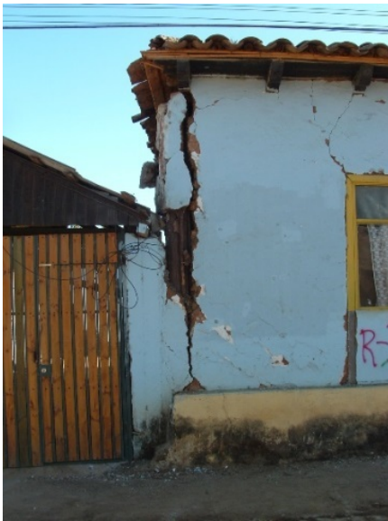
Figure 10. Separation between adobe walls after the 2010 Maule earthquake in the city of Curepto
