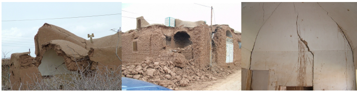
Figure 5. Partial and complete collapse of arched roofs: (a) Zarand Earthquake
