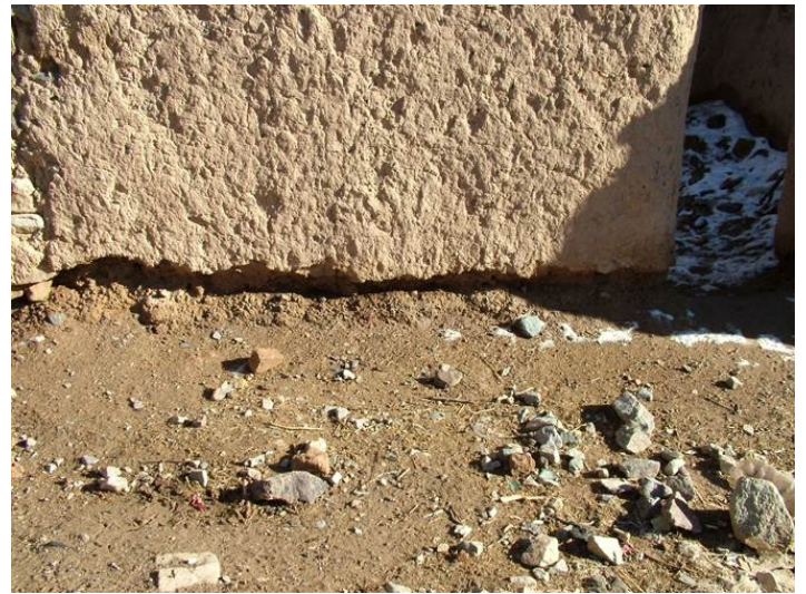
Figure 12. Wall slippage due to lack of proper foundation
