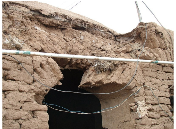
Figure 14. Common cracking around adobe arched openings in past earthquakes: (a) Zarand earthquake (2005), (b) Unknown, (c) shake-table tests by Bakhshi et al. (2009)
