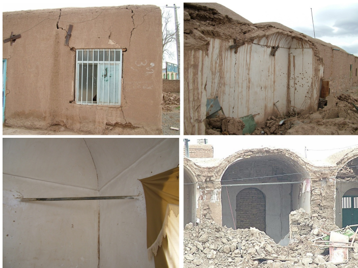
Figure 15. Using steel rods and welded steel mesh for enhancing the seismic performance of adobe walls in out-of-plane and in-plane directions: (a) Zarand Earthquake
