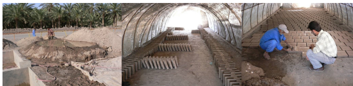
Figure 9. Construction of sun-dried, baked square and rectangular adobe blocks: (a) restoration of Bam Citadel by Hejazi and Mehdizadeh (2013)
