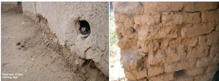
Figure 13. Deterioration of adobe walls due to weathering and lack of/improper foundation insulation
