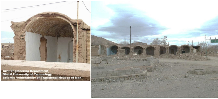
Figure 11. Out-of-plane collapse of non-load-bearing walls in barrel adobe roofs
