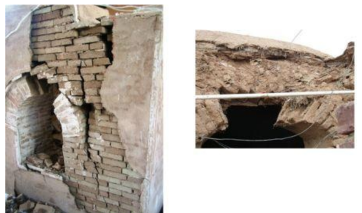
Figure 14. Common cracking around adobe arched openings in past earthquakes: (c) shake-table tests by Bakhshi et al. (2009)
