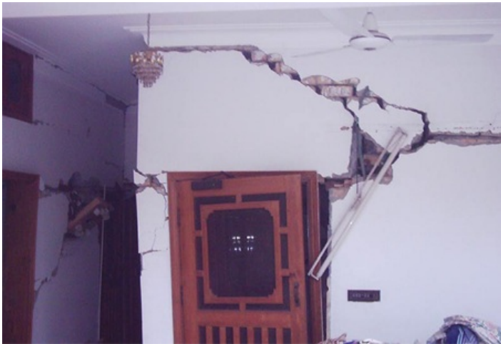
Severely damaged unreinforced brick masonry wall in Muzaffarabad during the Kashmir Earthquake of 2005 [5].
