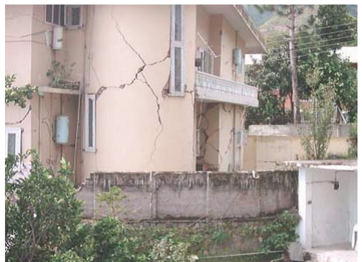
Typical scissor type cracks in a two story brick masonry house at
