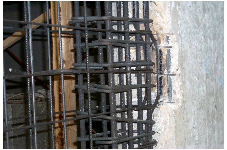
Seismic Strengthening - Connection of the Old and New Concrete (Welding of Rebars)
