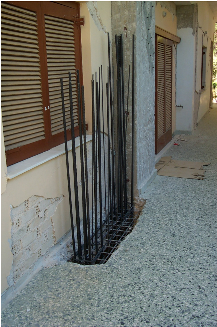
Seismic Strengthening - Extension of the New Shear Wall Through the Floor Slab
