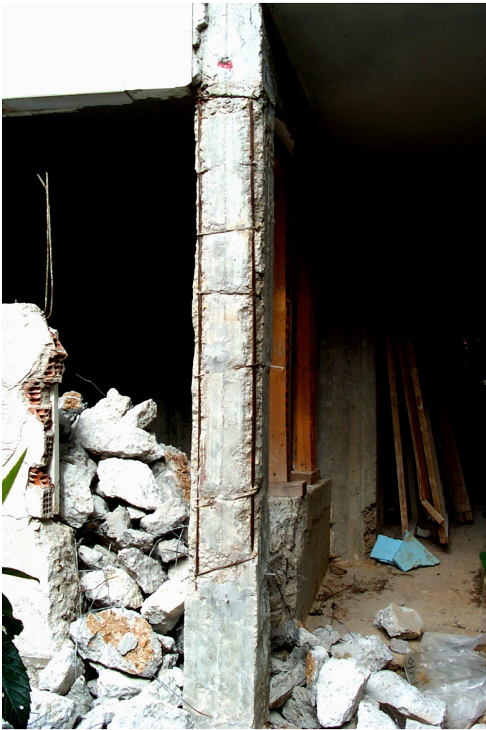
Typical Earthquake Damage to a Column of the Older 1960 Astructure (1999 Athens Earthquake)
