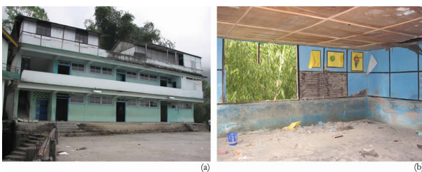
(a) Construction of additional Ikra type class rooms on third floor (on right side) of a reinforced concrete school building, and (b) damage sustained by the walls of the class rooms during 18 September 2011
