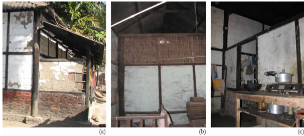
(a) Details of mud-dung plastering on walls, (b) and (c) arrangement of internal walls.
