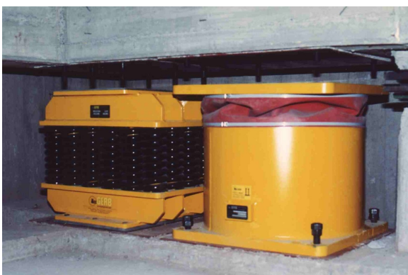
View of System of Isolation in BSI Building
