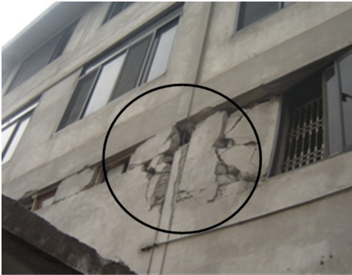
Building being supported by infill walls after failure of column
