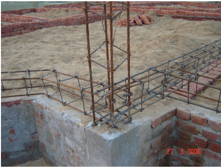
Beam reinforcement hooking into column reinforcement. Also note inadequately large spacing of stirrups in the beam and column, and no stirrups in beam-column joint.
