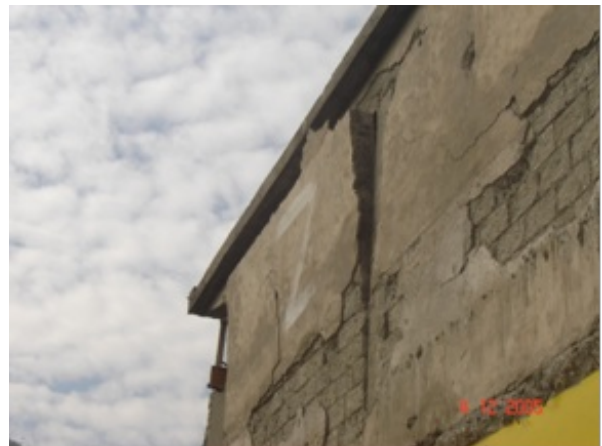
Onset of out-of-plane collapse of infill wall
