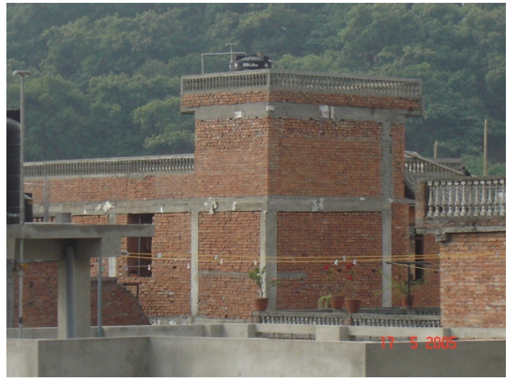
Missing columns in top storey
