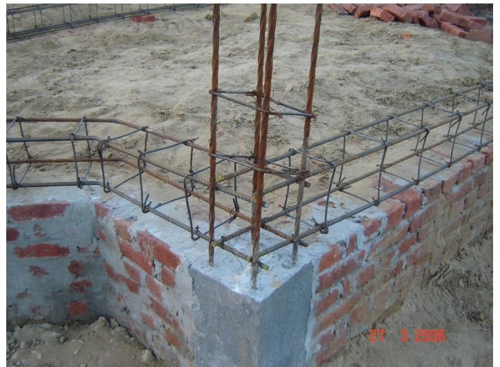
No anchorage of beam bars in column
