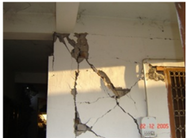
Failure of column due to shear imposed by infill wall
