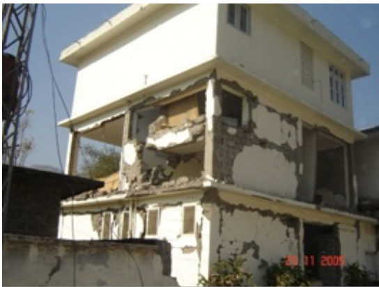
Onset of development of soft storey mechanism at 1st floor level
