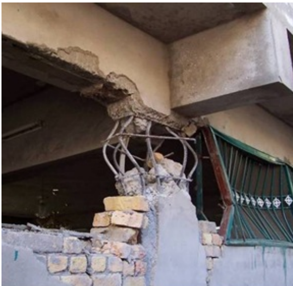
Short column due to partial height
