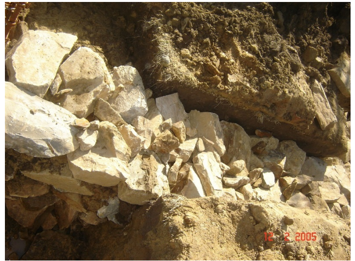
Constructing toe wall for tie (at plinth level) beam in stone masonry
