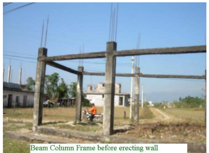
RC frame ready to receive infill walls. Note that there are no horizontal ties protruding from the columns to prevent the infills from
