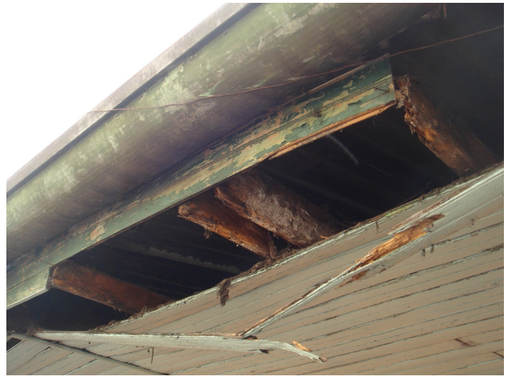
Rotten beams of the wooden roof construction.
