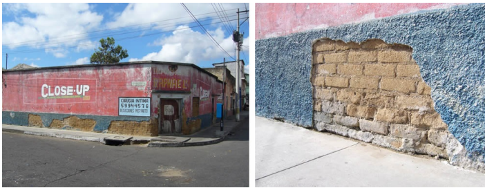
Spalling of plaster due to ascending moisture in the adobe walls (Guatemala City, Zona 7).
