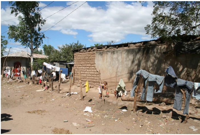
View from the road. The exterior plaster on the left side has fallen off due to the lack of eaves.
