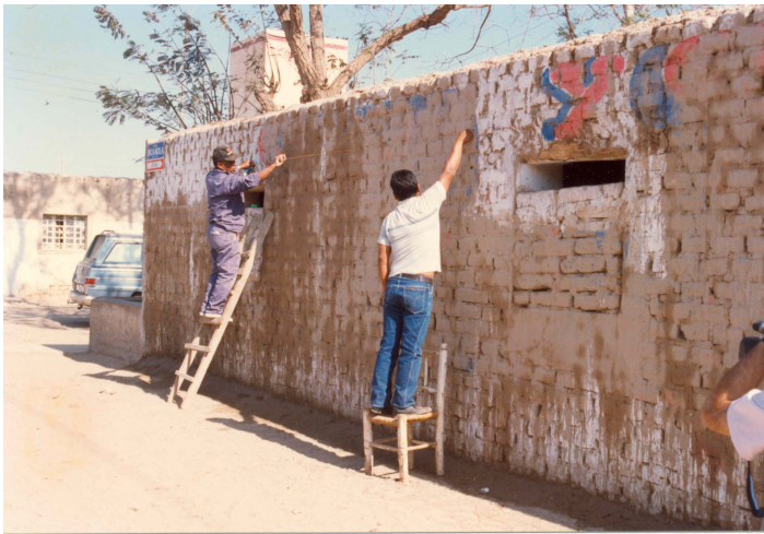
Reinforcement of existing house of Fig. 19 in Ica, in 1998. Workers mark position for horizontal strip.
