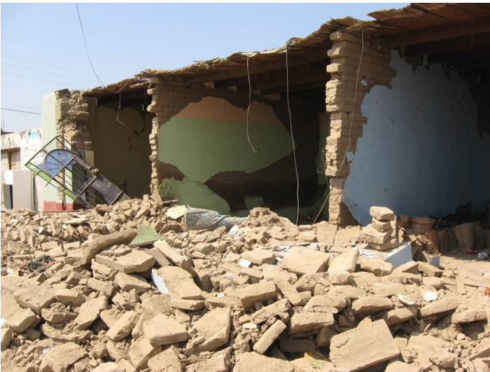
Collapsed houses in the same block as the reinforced house of Fig. 19, after the 2007 earthquake in Ica.
