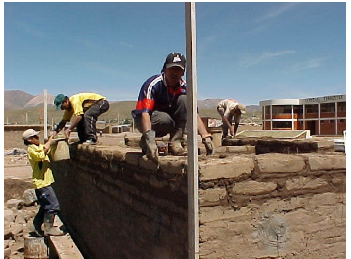
For new houses, check the width of joints and use connector wires in the joint
