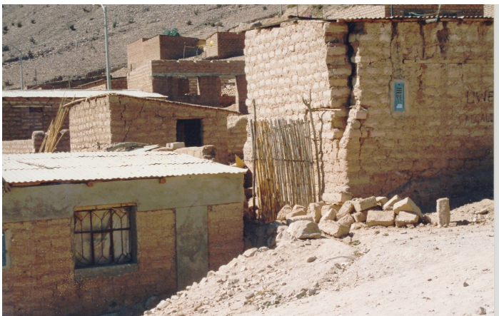
Inspection after 2001 Earthquake in Moquegua: reinforced house without damage and neighboring unreinforced house with severe damage
