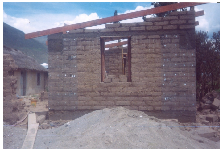
Strips of wire mesh nailed to the corners, and wood collar beam.
