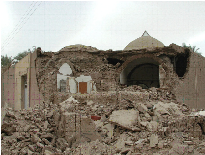
Key Seismic Deficiency: walls are not tied to roof, and can move out-of-plane in an earthquake
