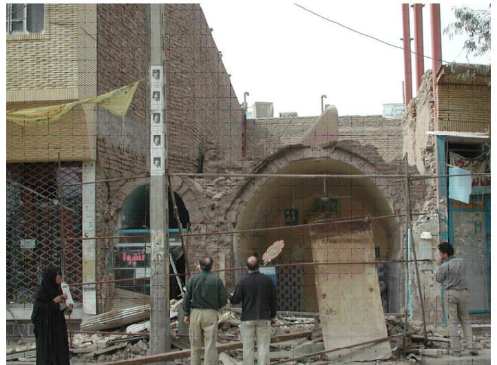
If walls can be kept in-plane, building typically survives. Adobe
