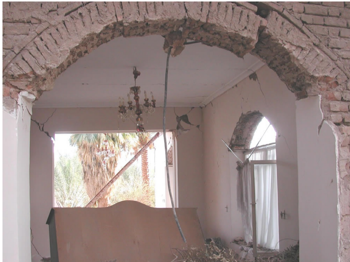
Bam earthquake: Damage to a traditional adobe house. Non-bearing walls collapsed, bearing walls are still standing
