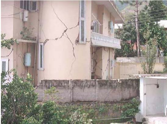
Figure 9. Typical scissor type cracks in a two story brick masonry house at Muzaffarabad, Kashmir [4].
