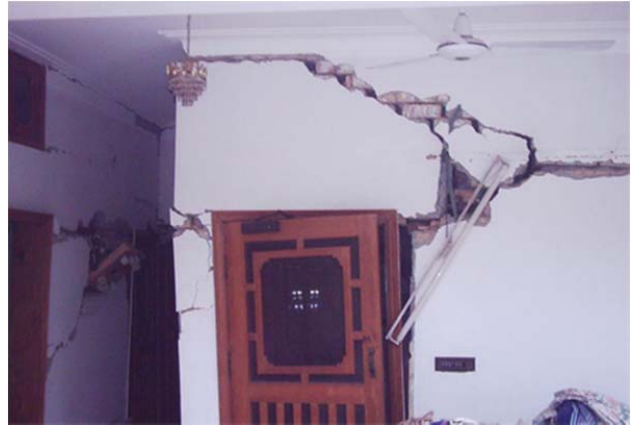
Figure 10. Severely damaged unreinforced brick masonry wall in Muzaffarabad during the Kashmir Earthquake of 2005 [5].
