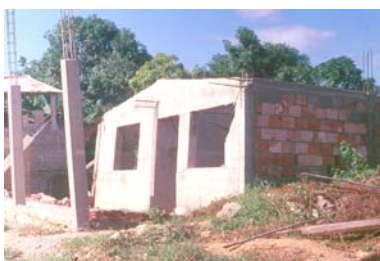
Figure 6: A Photograph Illustrating Typical Damage (1997 Cariaco earthquake)
