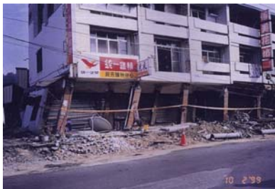
Figure 6A: A Photograph Illustrating Typical Earthquake Damage
